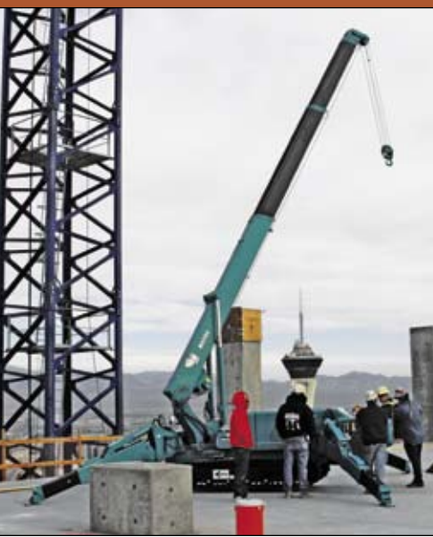
The Maeda mini-crane helps crews access areas of the roof inaccessible to tower cranes.
